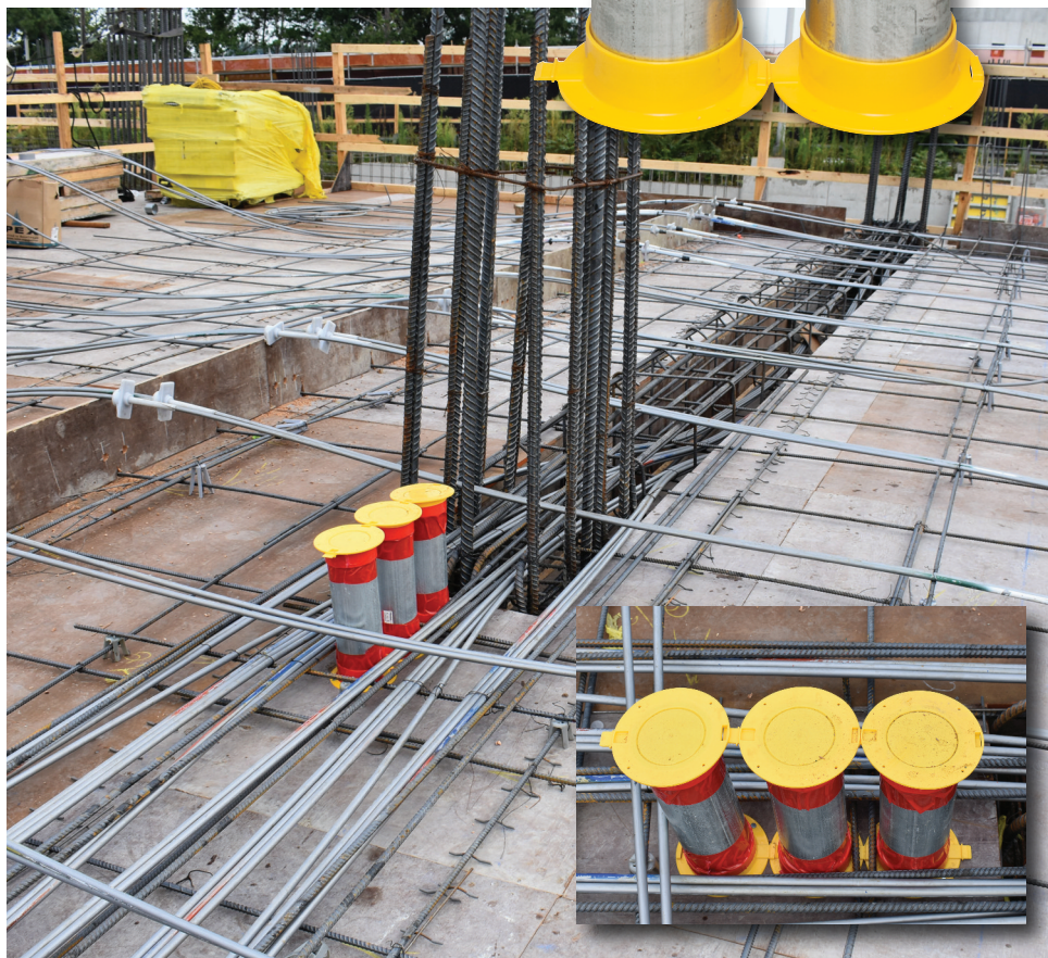
Three EMT400CFT bushings coupled together in commercial, six-story poured concrete slab.
